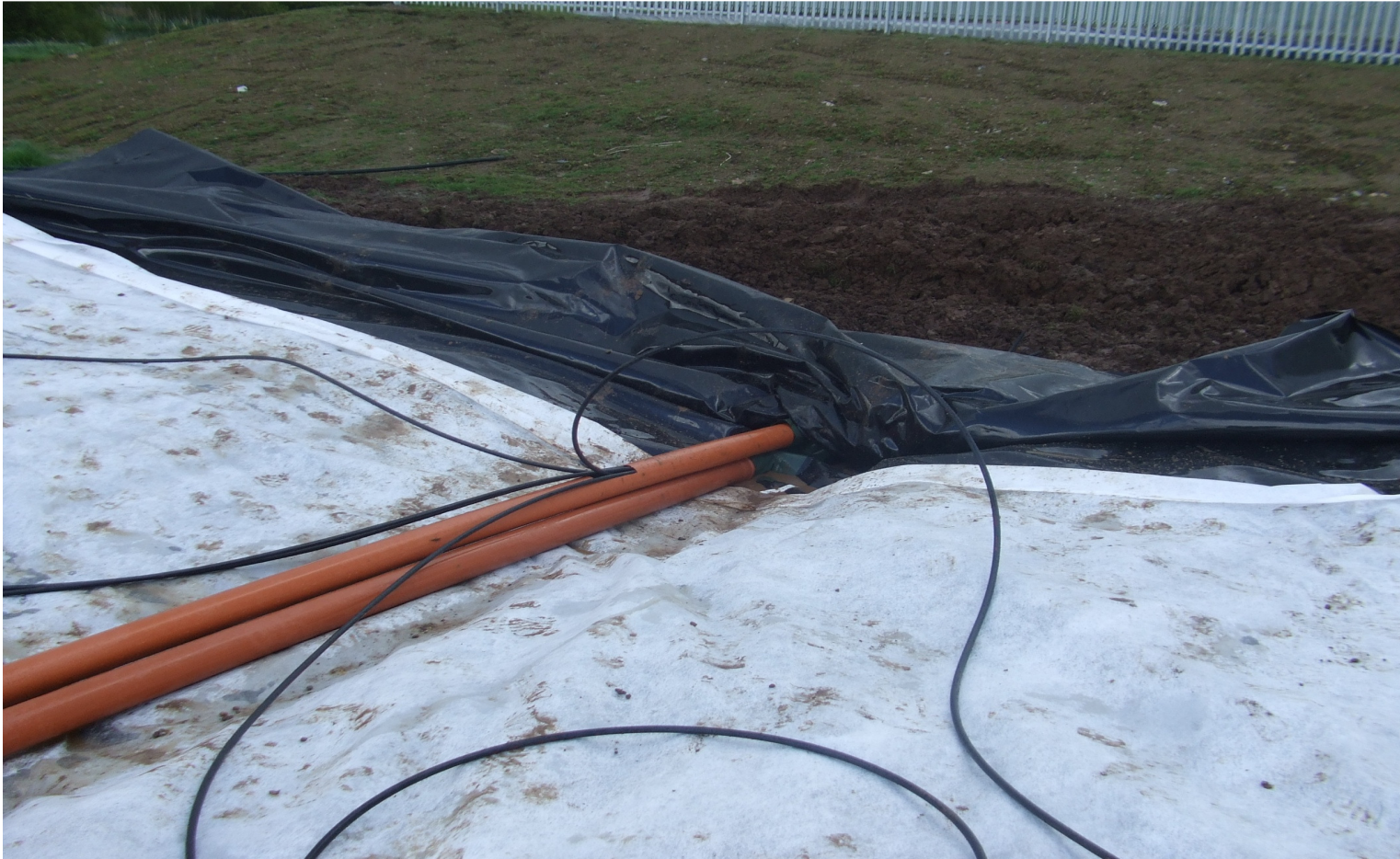
Effluent collection pipes exiting the liner at the base of the filter
