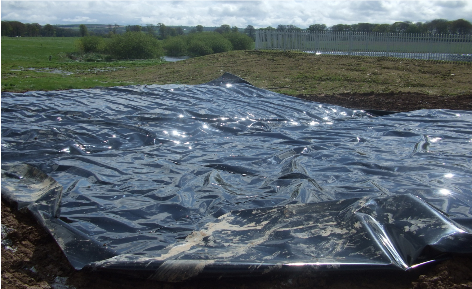
Liner to collect effluent at the base of the filter
