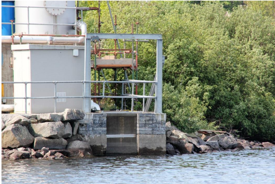
Figure 2.3 Screen at the abstraction point of a surface water source (Photo taken at test site of Chapter 5).
