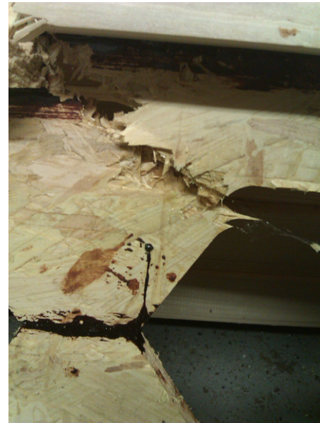
Fig. 8. Tension failure at corner of opening.
